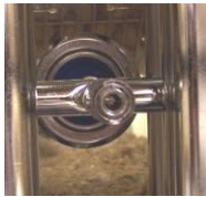
No water valve in place
