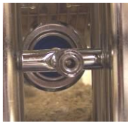
No water valve in place
